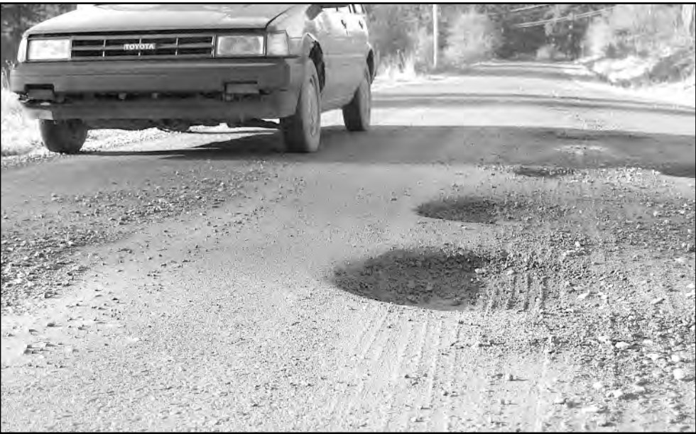
POTHOLES FOR THE COUNTING: Potholes such as these will be included in the second annual pothole count, set to run on Salt Spring until February 18.
