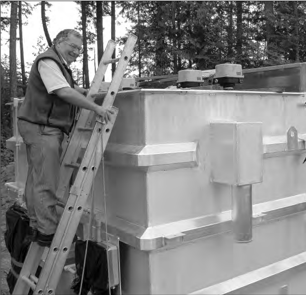
PHOTO BY SEAN MCINTYRE Trevor Hutton inspects the island’s newest piece of machinery. The dissolved-air flotation (DAF) unit is one of the pieces needed to complete ongoing work to upgrade the Beddis-Fulford water treatment plant.
